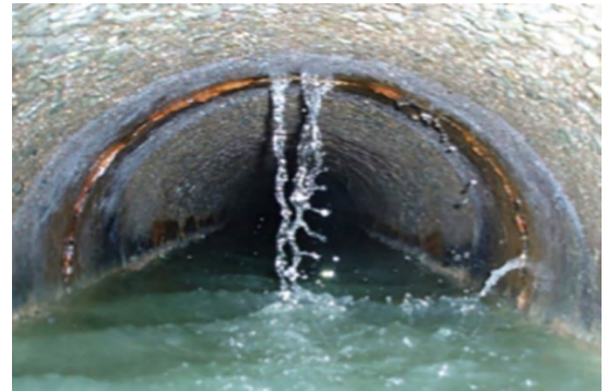
FIGURE 3. Example of Sanitary Sewer Infiltration
