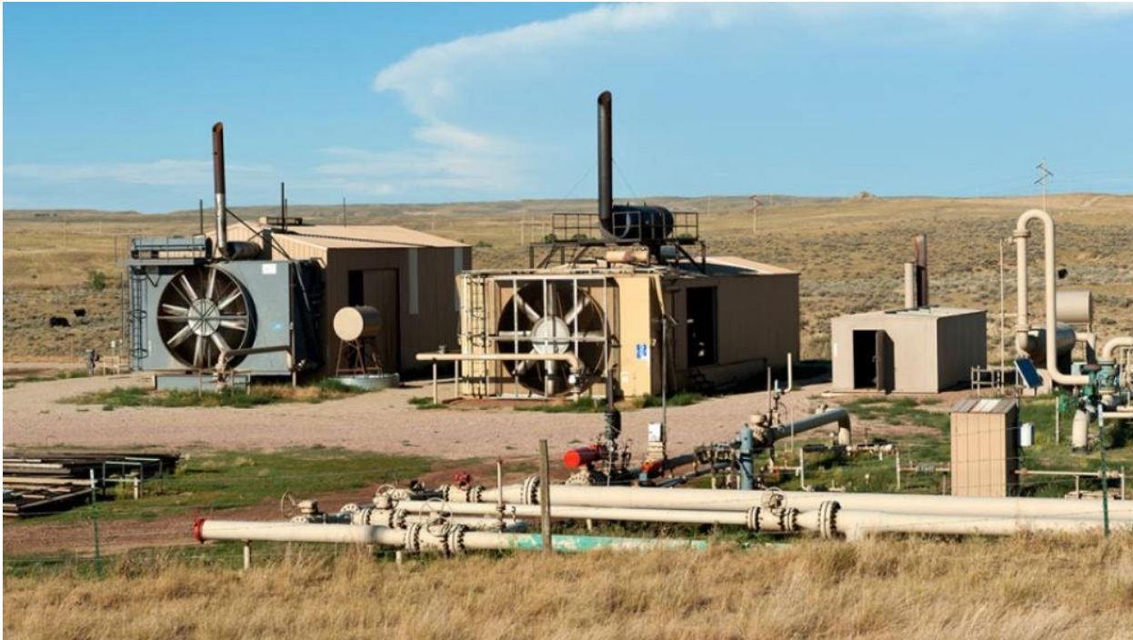
Process Photo no. 3 – Natural Gas Pipeline Compressor Station
