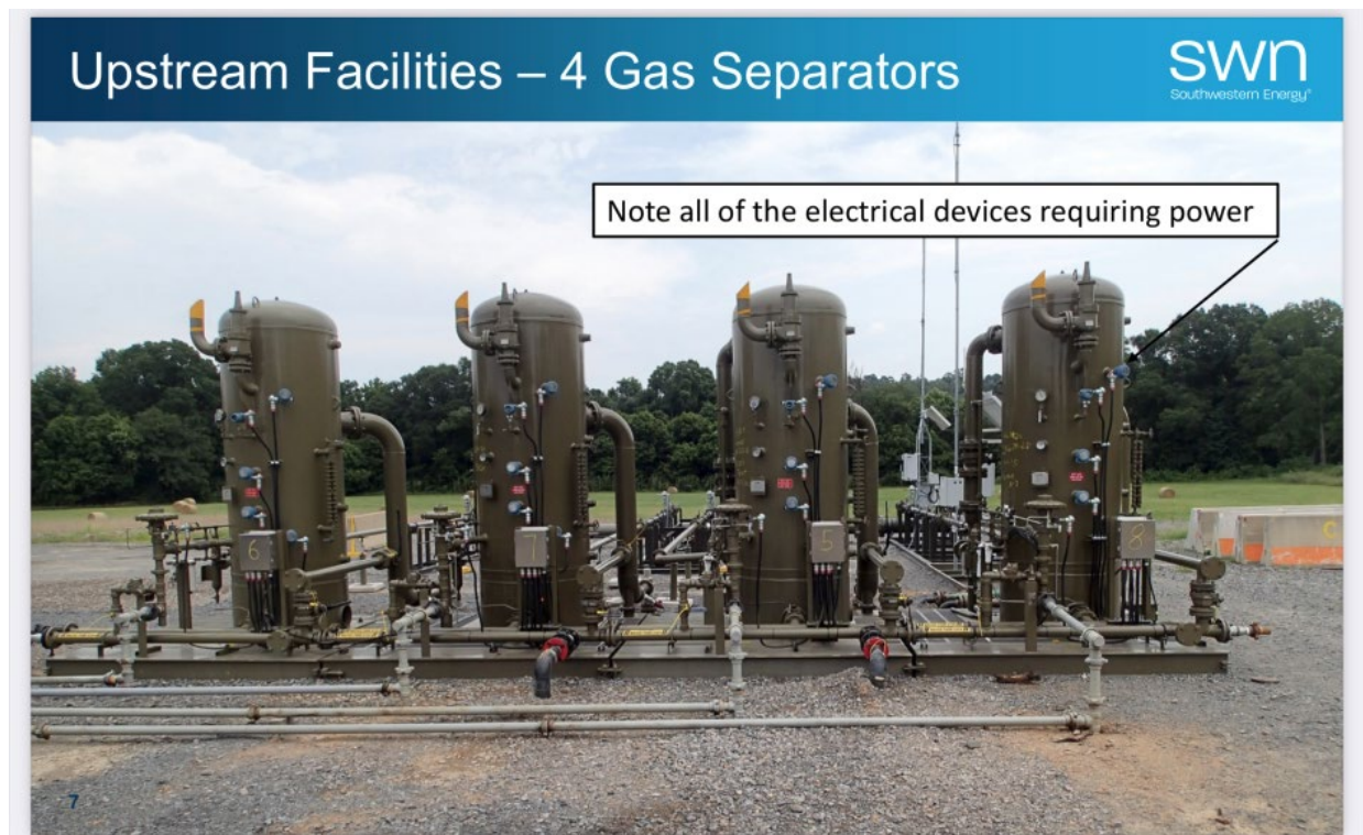
Process Photo no. 1 – Field oil and gas separation vessels layout and controls
